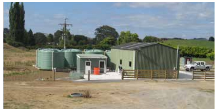
Piopio Water Treatment Plant.
