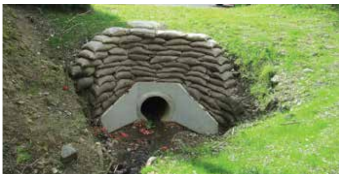
Rehabilitation work was undertaken on the inlet to the stormwater drain located on Butler Street.
