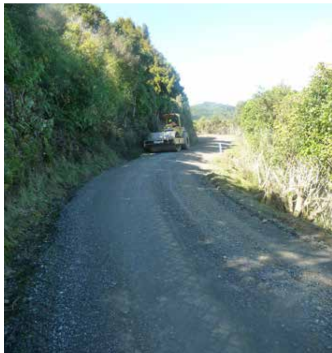
WDC's roading contractor Downers, carry out pavement rehabilitation works on a rural road in the Waitomo District.
